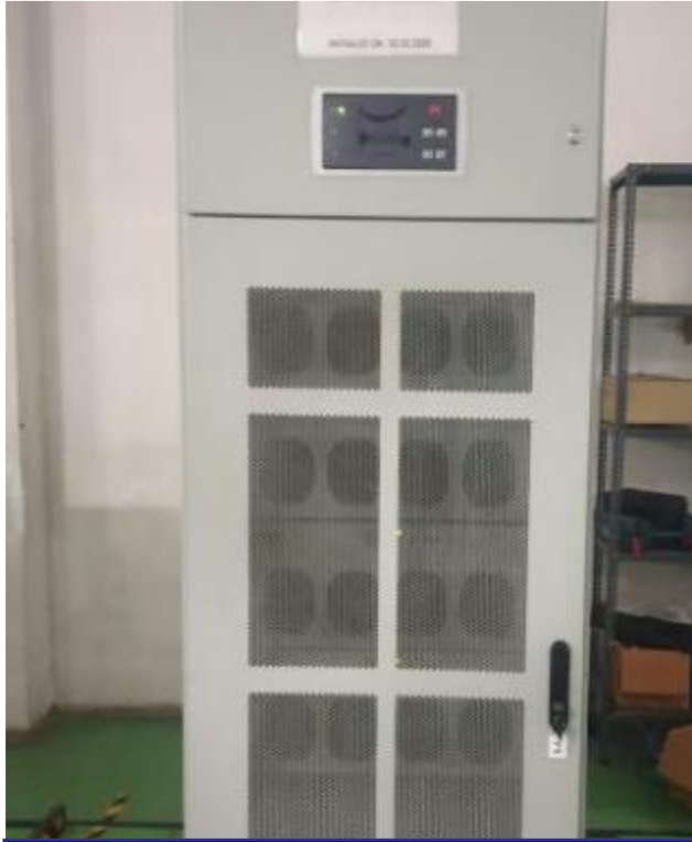
Active harmonics filters were installed to improve power quality
